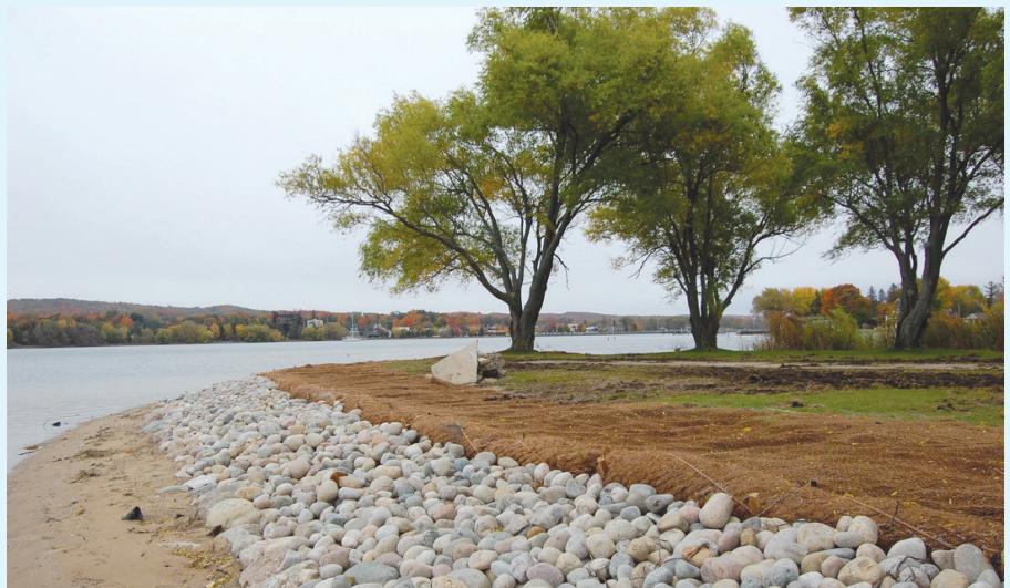
In the spring, the LCA will install native plants throughout the coir logs and the woven coir blanket. As these plants become established, they will “creep” toward the water’s edge.
